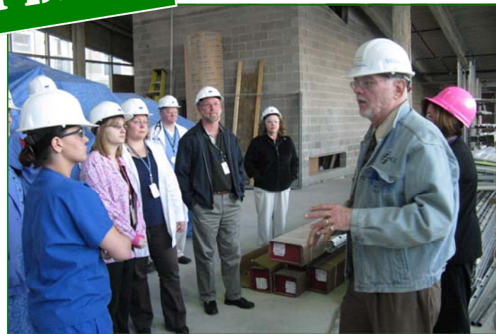
Robert Hawks, Mercy Hospital's Construction Project Manager, leads a group of associates on a tour of the new Emergency Department addition that is set to open in the spring of 2010. Preview tours began in mid-November and will continue over the next few months.
